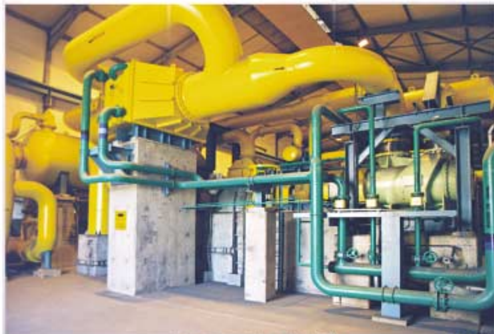
Multistage processgas vacuum pump-set, with interstage water cooling, 50 000 m 3 /h, final vacuum 100 mbar
